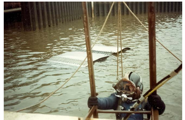
Diver Scott Anderson, of Logan Diving & Salvage, entering the water to install a 36" three piece extended range clamp on a failed pipeline in Georgia's Savannah River.
